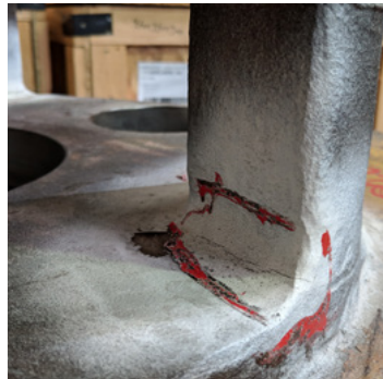
Carrier Pillar Cracking
